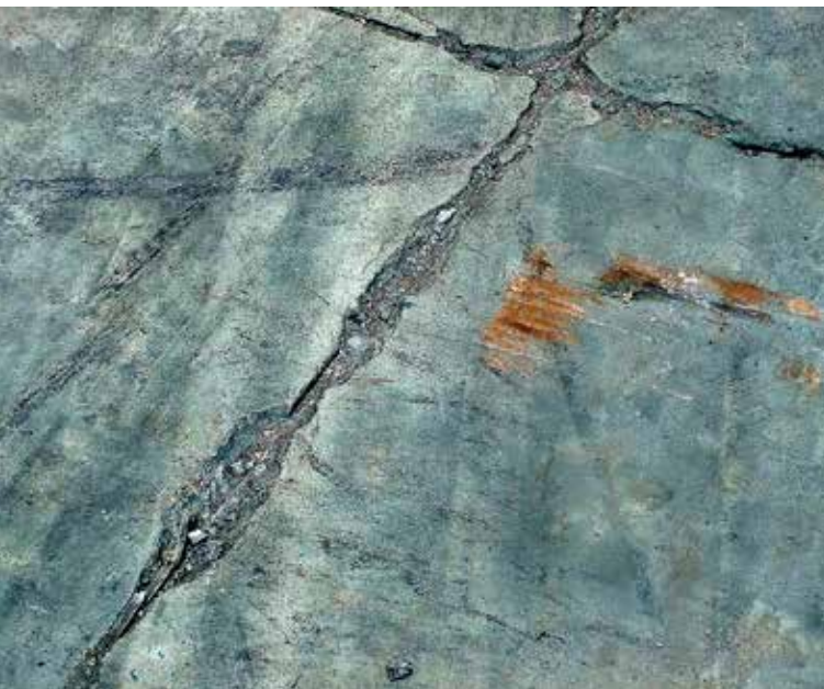
Examples of joint spalling in concrete floor slabs.
