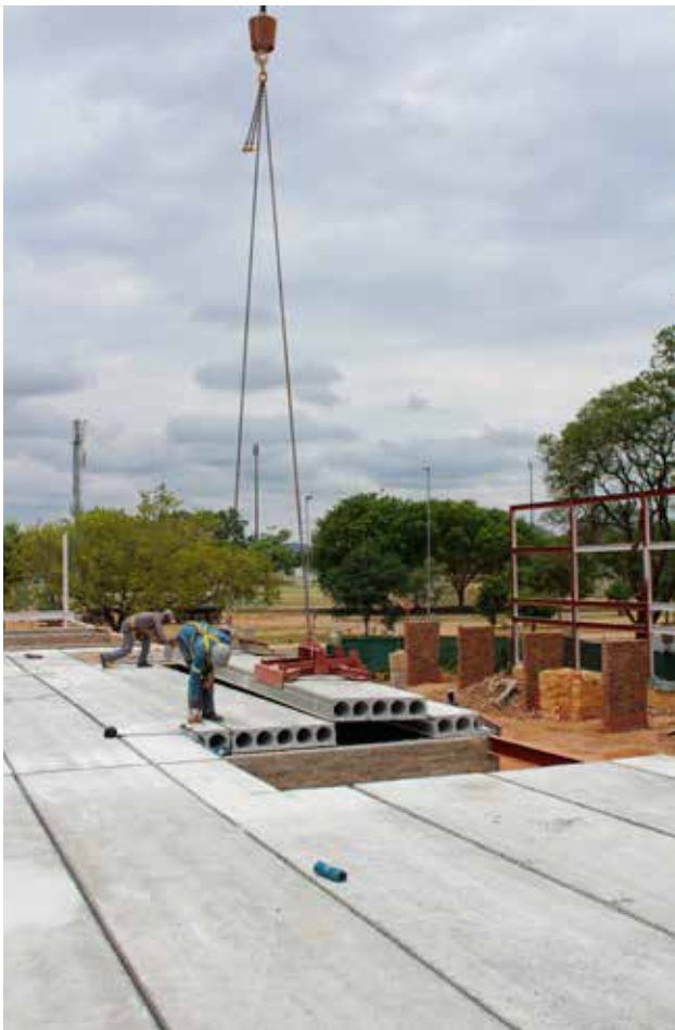
More than 90 hollow-core slabs, each 8 m x 1, 19 m, were delivered to site from CoreSlab's state-of-the-art factory every day in line with the works programme.
