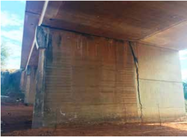
The badly cracked bridge pier before repair.
