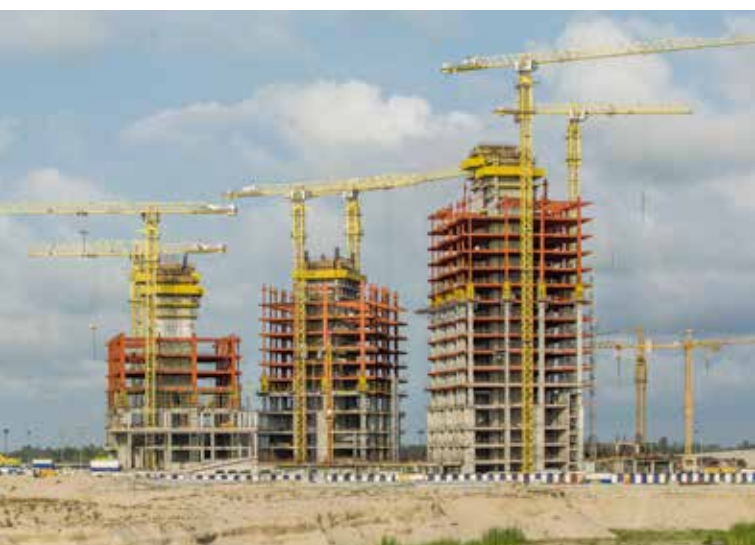
Since December 2016, work has been in progress on three residential high-rises (Orun Tower, Oban Tower and Zuna Tower).
