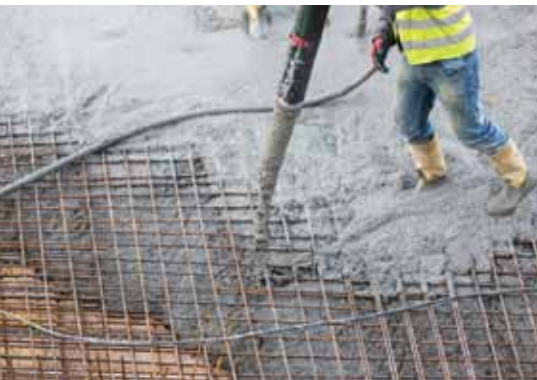
A superplasticiser gives a nice pump pressure maintains slump retention for quite some time.
