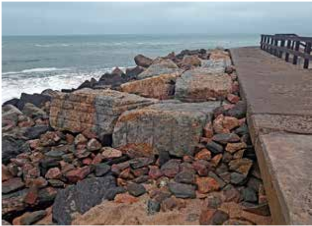
Swakopmund Mole retaining wall, with extra-heavy rock rip-rap. Pic supplied by Oliver Rust.
