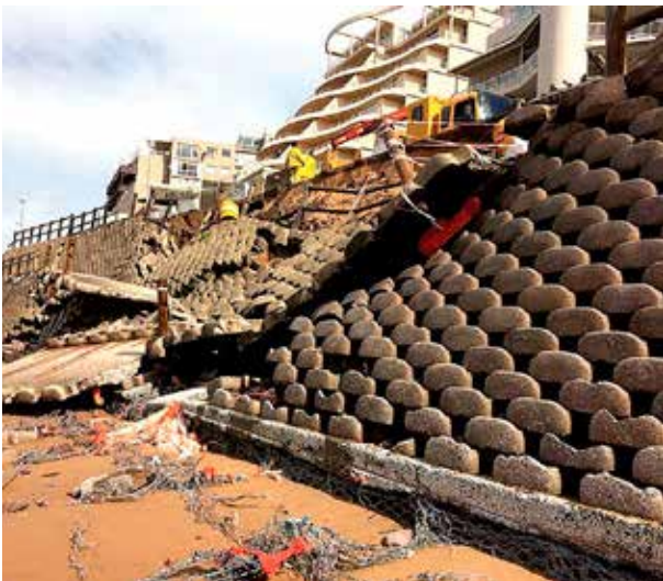
Umdloti beach failure.
