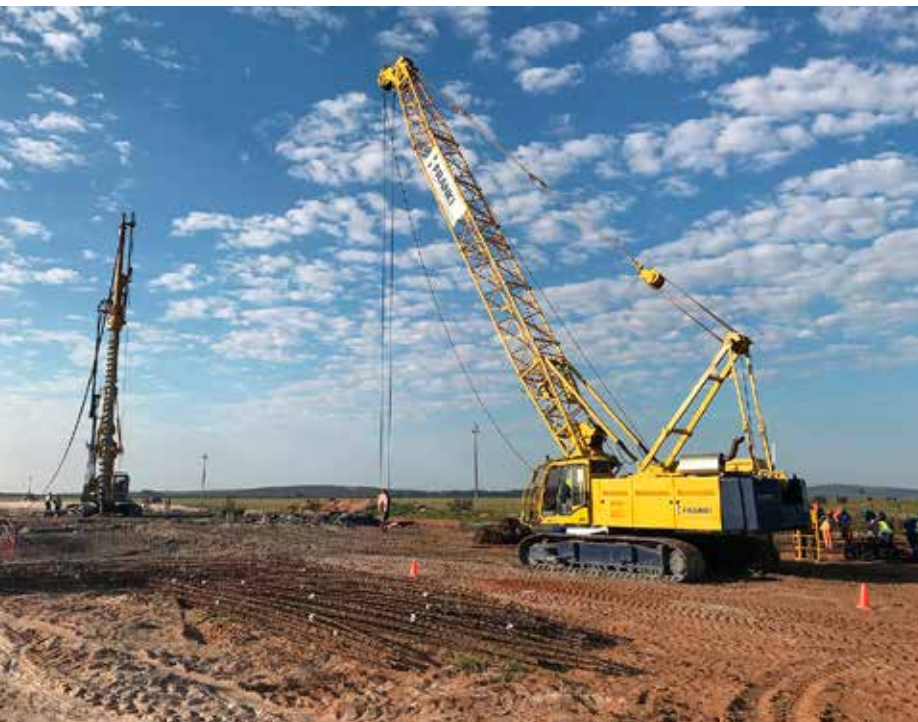
The geology of the site consists of windblown sands for around 0.5 – 1.0 m below natural ground level
