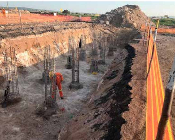
The test pile results proved the alternative methodology was correct and working piles were installed.
