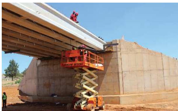
The new bridge over the Mankgatle River is one of two large structures along the route.
