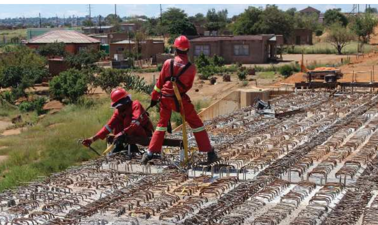
Lonerock Construction completed the bulk of the complex structural work ahead of the roadworks.
