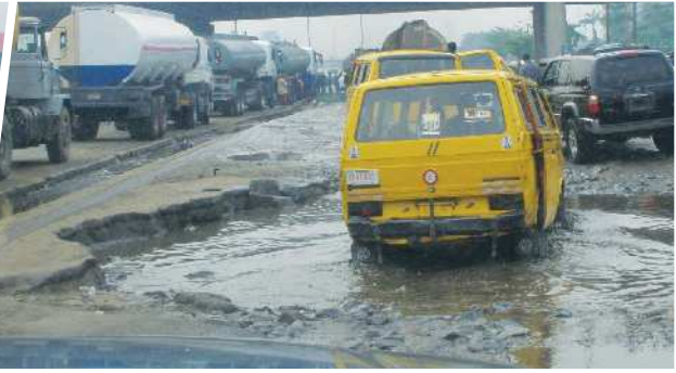
Catastrophic pavement failure due to unacceptable moisture conditions combined with overloading. (Looking for good in Lagos, 2011)
