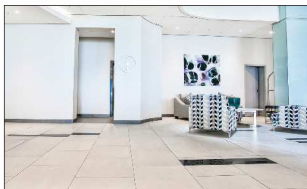
A smooth and level surface reduces lipping of large format tiles as evidenced at the Pearls of Umhlanga development.
