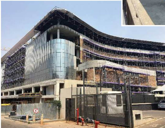
Perlite and cement composite lightweight concrete screeds going into the new Exxaro Head Office building in Centurion. The material was mixed with 42,5N cement on site, placed at 150 mm thick and will have a typical cured density of less than 500 kg/m 3 .
