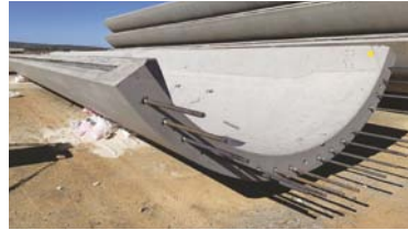
CHRYSO Southern Africa is adding value to the precast concrete segments used to construct the 100 metre tall wind turbine towers
