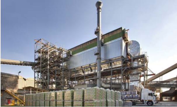
AfriSam has taken a number of approaches over the past 20 years to reduce its carbon footprint
