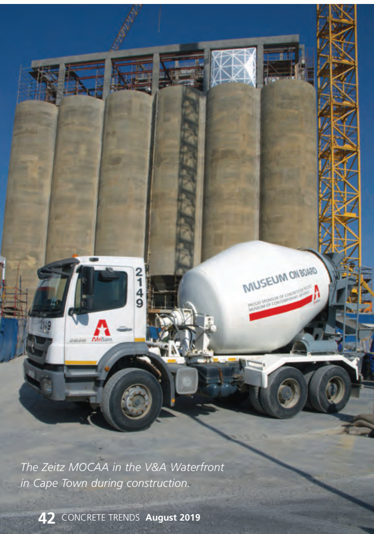
With evidence of the longevity and potential of its products on display in infrastructure across southern Africa, AfriSam's presence is widespread.
