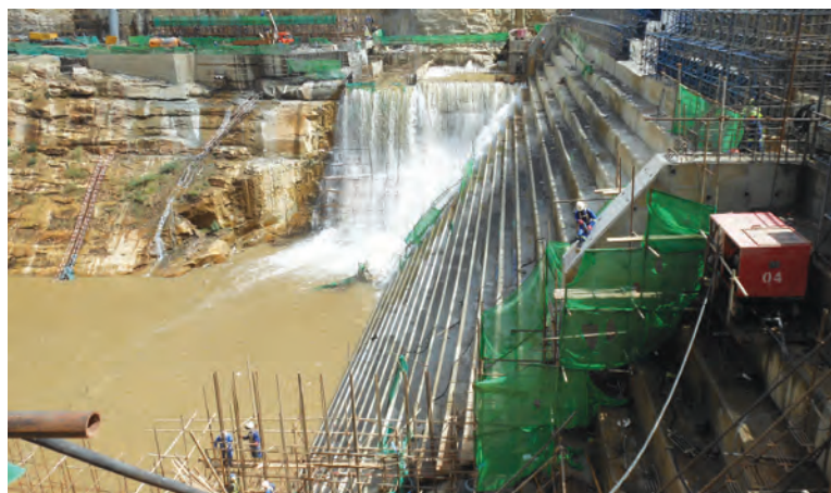
The innovative Lafarge products provided the solution for the RCC and CVC concrete.
