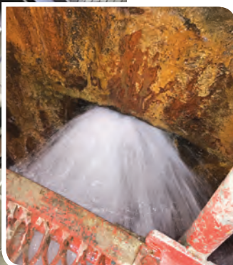
Major Water penetration through holes in the shaft wall.
