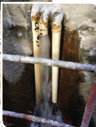
Major water ingress contained to a single point using Kryton plug.
