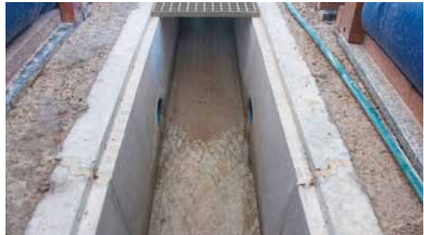
Sea water drains from the abalone tanks into a channel from two outlet feeder pipes.
