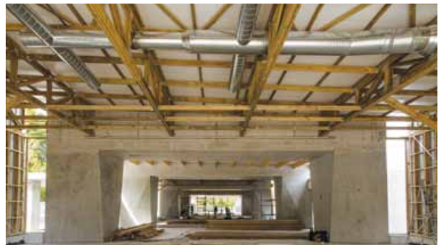
One of the roof-truss assemblies which was mounted between two in-situ roof beams.
