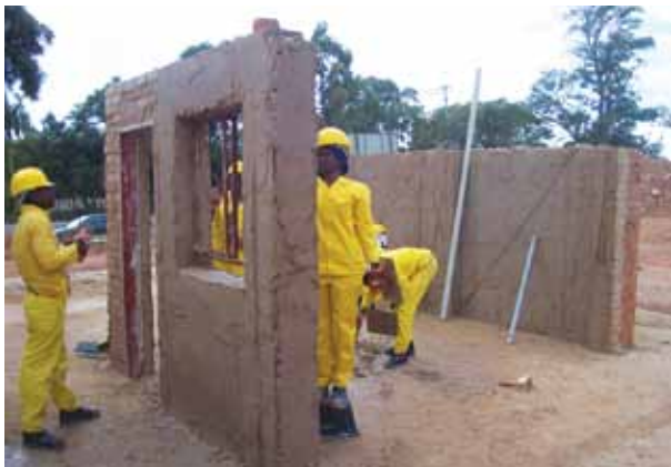
All training for the various building trades is undertaken in designated workshops or training areas
