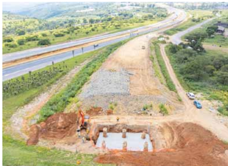
Important road projects in KwaZulu-Natal has also brought some relief to contractors and the supply chain
