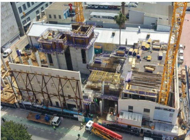
The supported heritage facade – overlooking Bree Street – takes pride of place on Concor Western Cape’s 16 On Bree site in Cape Town city, behind which the lift shafts rise quickly skyward
