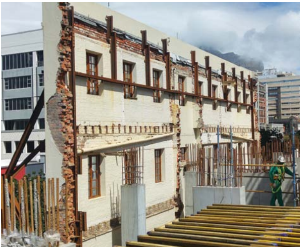
Viewed from inside the site, the specialised steel bracing is visible on the 200-year-old facade wall that has been preserved for heritage
