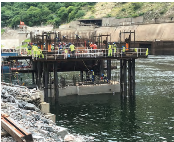
The first concrete pier set to float, which has a total length 5 metres.
