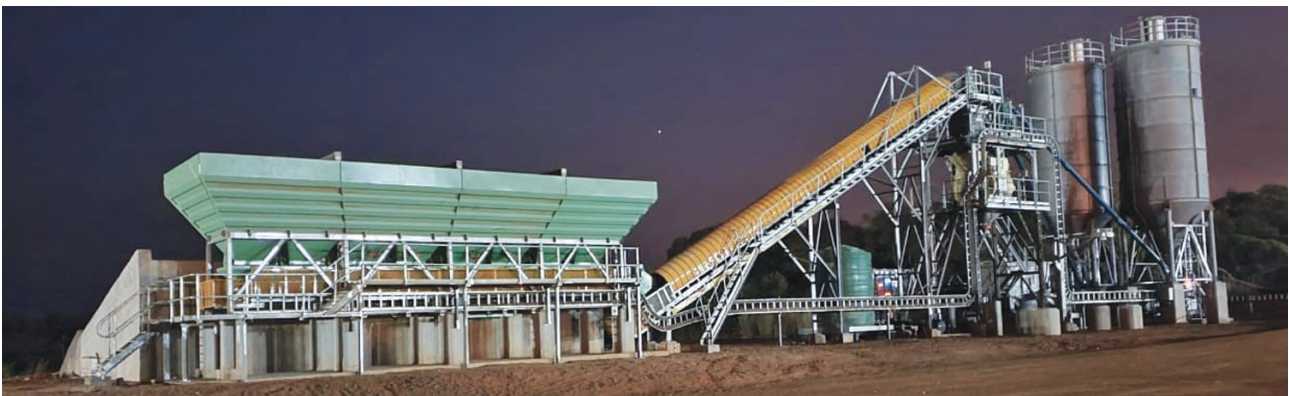
A night scene at a typical batch plant
