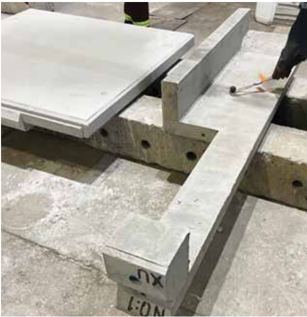
One of the top level panels cast with a recess to fit around the concrete beam at the top of the building.
