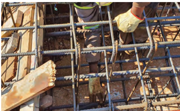
The company was appointed to undertake parts of the in-situ concrete work on a new 30ML reservoir in Selcourt
