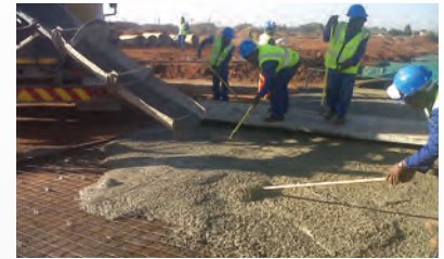
Spreading of wet concrete, note bridge to prevent walking on concrete or the steel mesh
