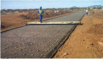
A section ready for concrete, three sections of 100 m 2 per day can easily be achieved by each team
