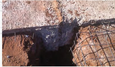
Anchor beams with soft board separation
