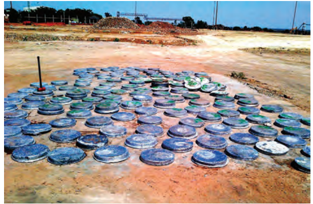
Decontamination of lead ingots
