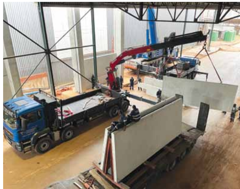
A precast panel is offloaded prior to installation in the strip section.
