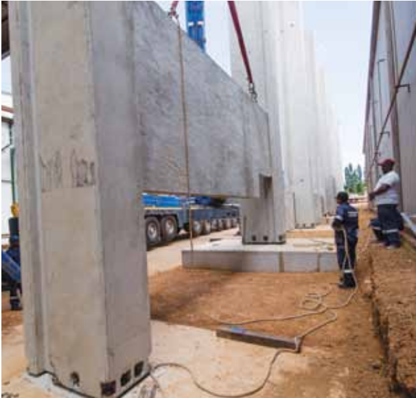
A precast concrete panel is installed between columns in the narrow strip section.
