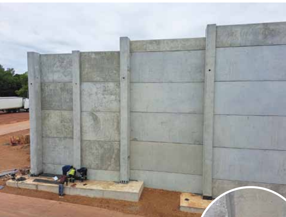
Some of the fireproof sealing which was installed on the panel-to-panel and panel-to-column jointing.
